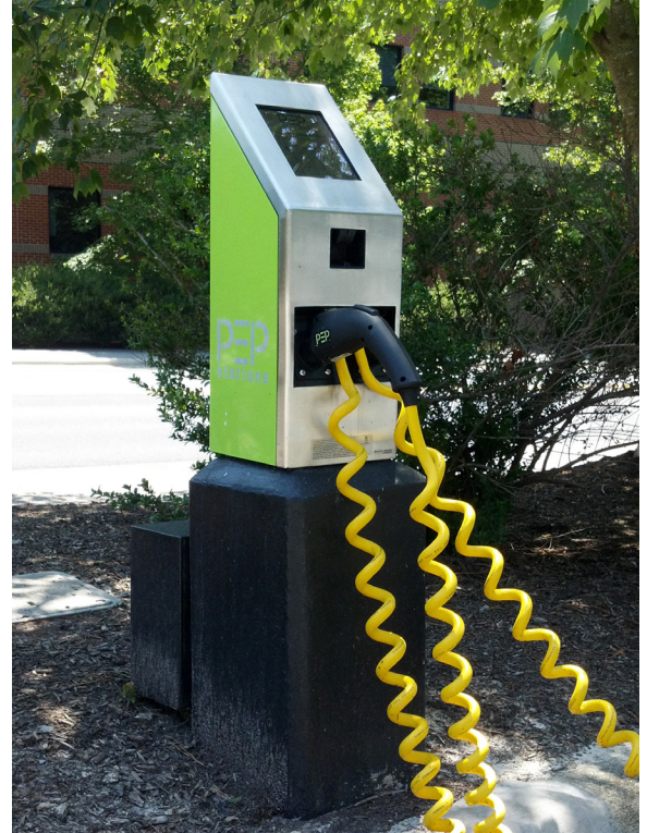
Example of charging station installed at Pentair's Sanford, N.C. manufacturing facility.
